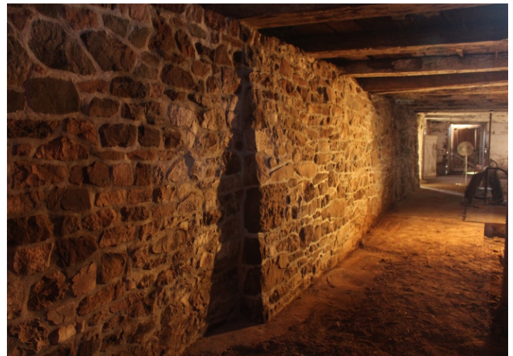
Above, an HGAC barn grant helped to pay to rebuild the battered monolith and back wall of the Mulligan Barn #262.
