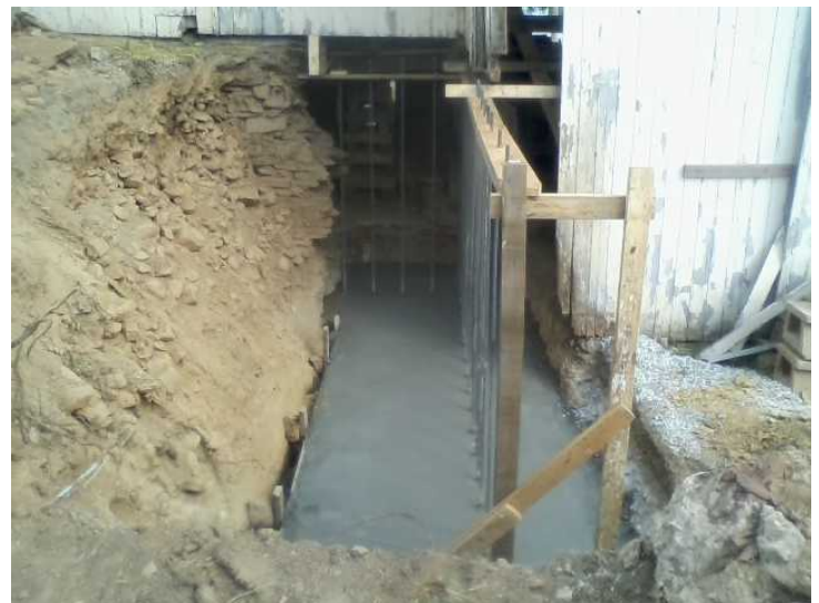
Below, an HGAC barn grant helped to pay for replacing the foundation footer on the Stricker Barn #240.
